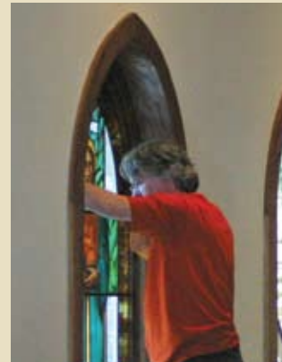
The windows were installed over Christmas break so that the students' chapel program would not be interrupted.
